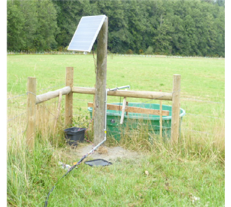
Solar water pumps
