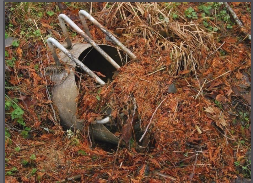
Blocked outlet to control structure
