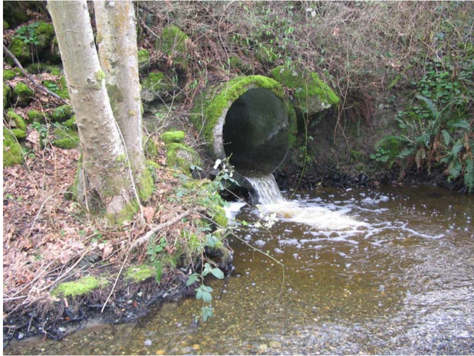
Perched culvert, Franklin Road, Little Fisher Creek
