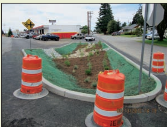
This raingarden, located at the Hazel St/Anacortes St/North Cascades Hwy. intersection will add aesthetic appeal to the neighborhood in addition to providing numerous environmental benefits.
